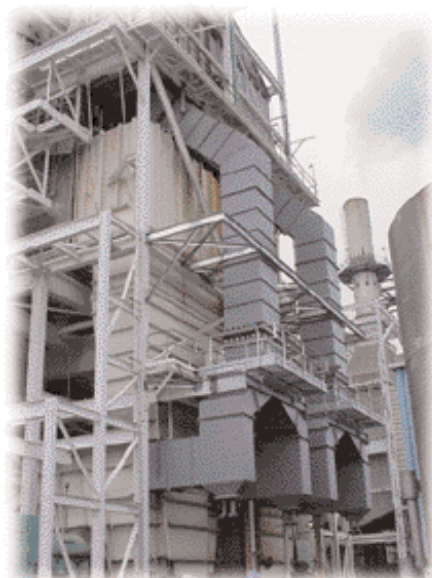
Typical power plant IFGR installation.
